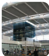
Omni antennas at airport for PMR and TETRA
